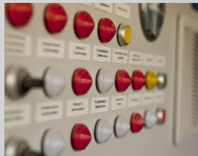
Schaltkasten THS-MV Switch cabinet THS-MV
