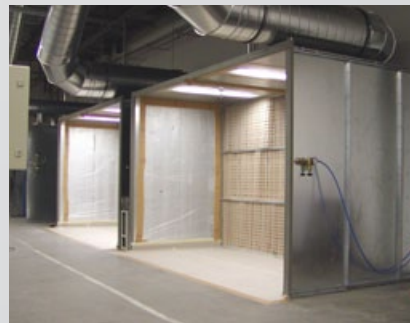
Fester Vorbau 1,5m tief mit EX-Leuchten Fixed wall mounting 1.5m deep with expl.-protected lighting
